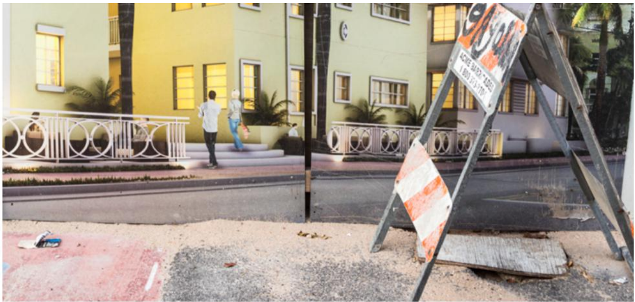
Anastasia Samoylova: Construction in South Beach, 2017 Image courtesy of the artist and Galerie Caroline O'Brien
